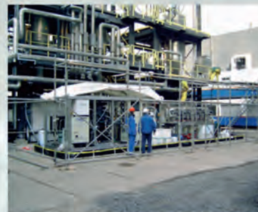
Pilot demo of soda crystallisation at AVR, Rotterdam
